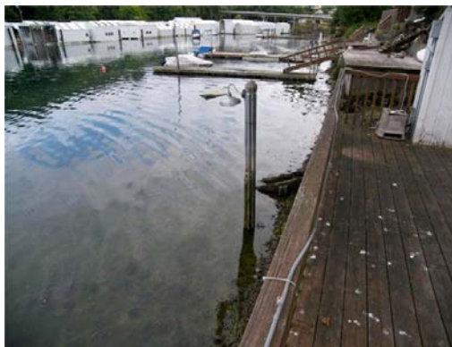
One of two pilings with electricity ready for your dock.
